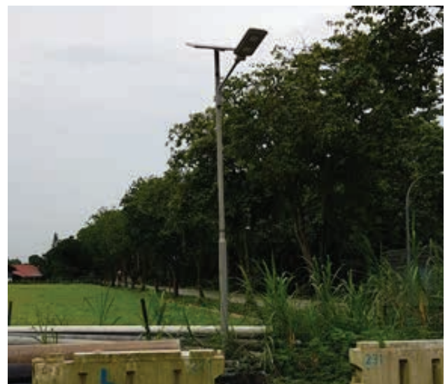
Solar panel lights at Ley Choon premises
